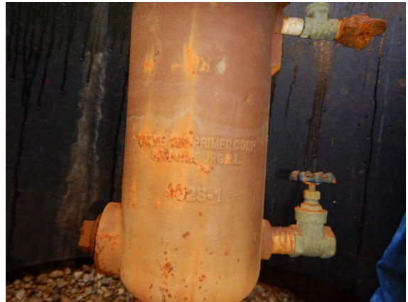
ARV 1350 Nottingham ARV With (2) Valves That Did Not Turn With Minor Rust Nottingham Erosion
