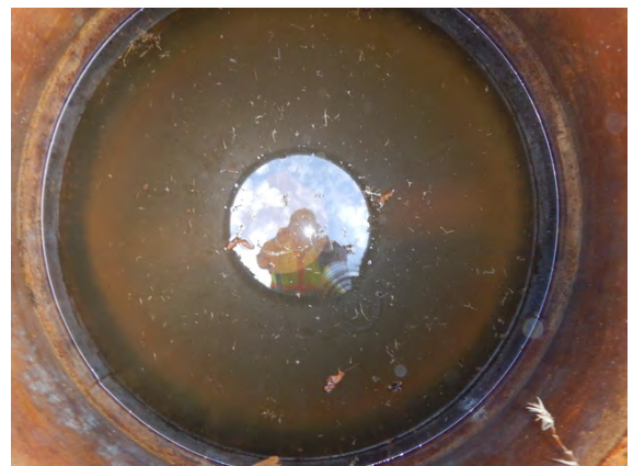
ARV 1300 Crossing Manhole Surcharged
