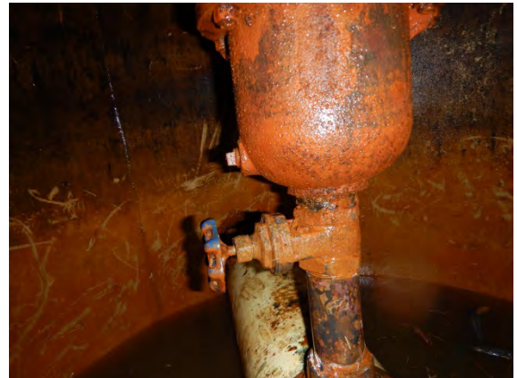
ARV 1300 Crossings Valve in Good Condition
