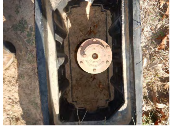
ARV 1291 Pilot Force Main Not Visible in Vault; ARV Operated While on Site, Valve Locations Capped
