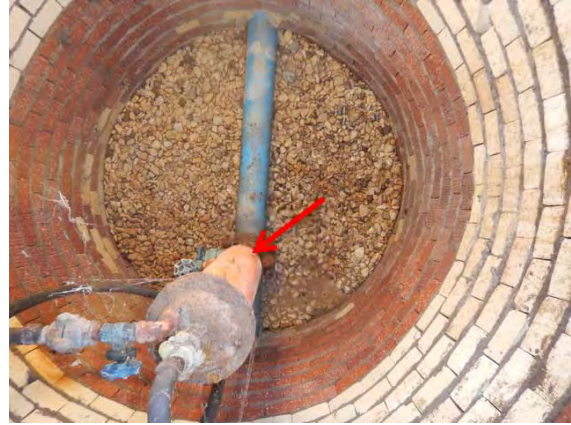
ARV 1310 Rustic Force Main Line Visible in Manhole; Moderate Corrosion on ARV Pipe Strap with Minor Rust on (3) Valves
