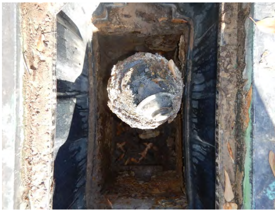
ARV 1260 Pilot Force Main Not Visible in Manhole; (1) Valve Not Operable
