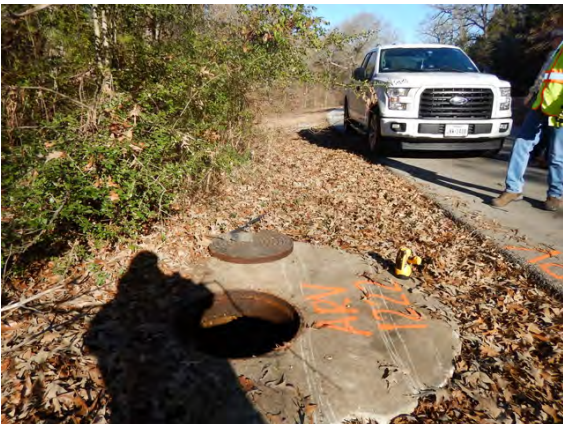
ARV 1222 Bellwood Area in Good Condition, Manhole Ring in Poor Condition
