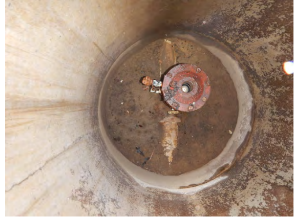
ARV 1221 Bellwood Force Main Visible in Manhole; Air Released While on Site
