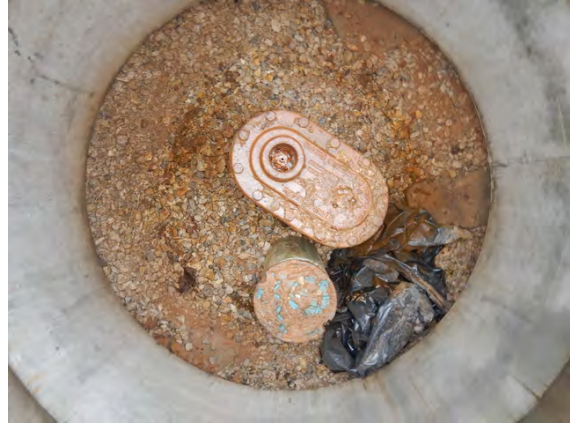
ARV 1330 Oak Creek Force Main Not Visible in Manhole; No Valves on ARV
