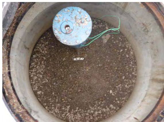
ARV 2060 Highways 31 West Force Main not Visible in Manhole; ARV Turns Properly but No Air Was Released
