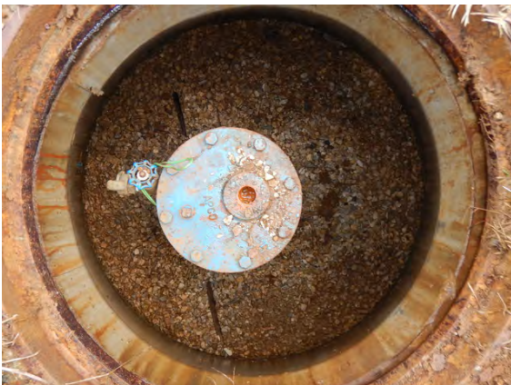
ARV 1231 Shackleford Force Main not Visible in Manhole; Top, Middle and Lower Valve Open to ½ Turn and Released Air
