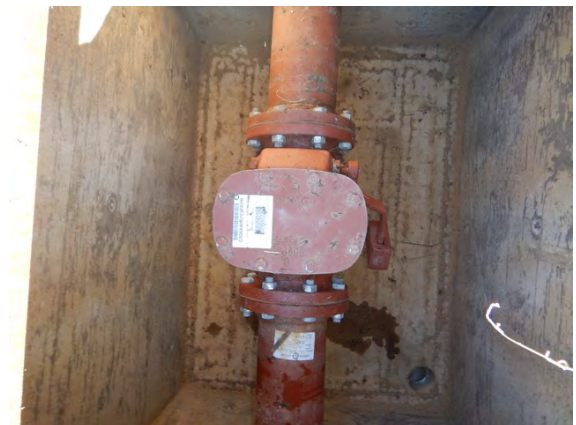
ARV 1271 Pilot Check Valve in Good Condition
