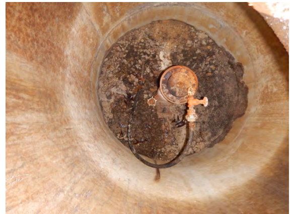
ARV 1222 Bellwood Top of Force Main Visible in Manhole; (2) Valves Operate With Minor Rust, No Air Released While Operating Valves
