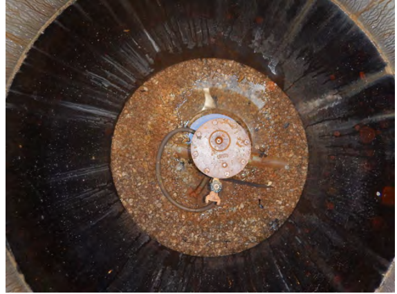
ARV 1350 Nottingham Force Main Crown Visible in Manhole; (2) Valves on ARV
