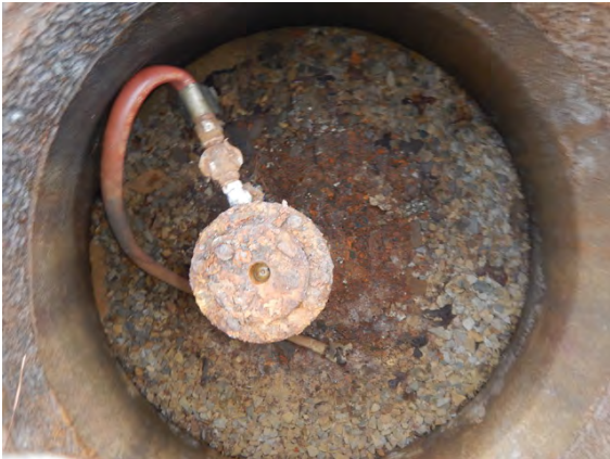
ARV 1230 Shackleford Force Main not Visible in Manhole; Minor Rust on Top and Middle Valve Opening Half Way, Moderate Rust on Lower Valve and Only Spins
