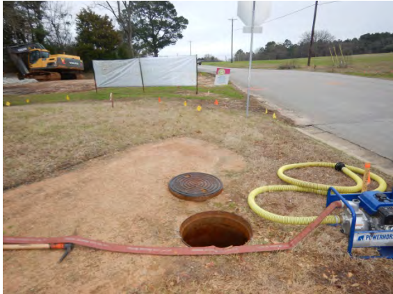
ARV 1300 Crossings Manhole and Area in Good Condition, Minor Corrosion on Manhole
