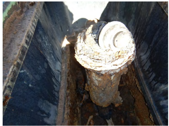
ARV 1260 Pilot ARV With Moderate to Severe Corrosion on Bolt and Body
