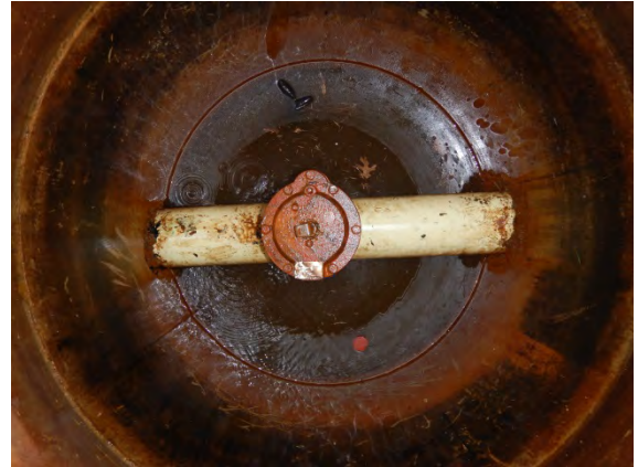
ARV 1300 Crossings Manhole Surcharged
