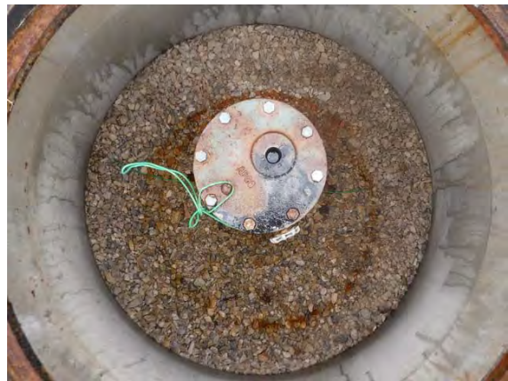
ARV 2050 Highway 31 West Air Release Valve in Good Condition, Valve Turns but No Air Was Released; Force Main not Visible in Manhole
