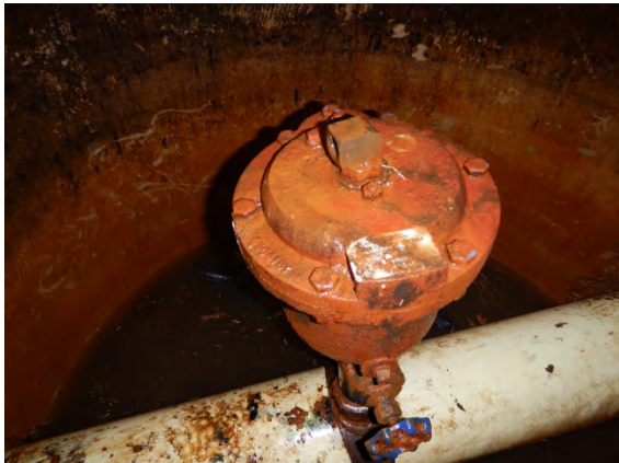
ARV 1300 Crossings Air Release Valve in Fair Condition
