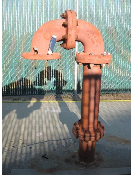
Corrosion on Ventilation Piping
