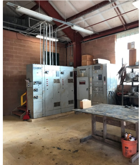
Electric Panel Inside Building Facing Northwest
