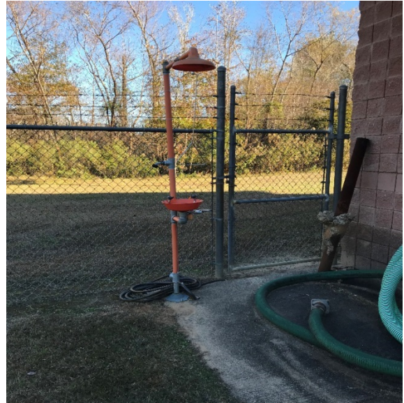
Eyewash Station Near North Fence
