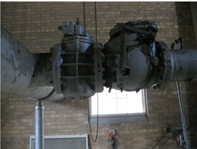
Grease Exposed on Valve. Flaking of Coating and Corrosion Observed
