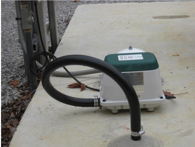
Air Compressor For Wet Well Aeration – Could Preferably Moved to Higher Ground
