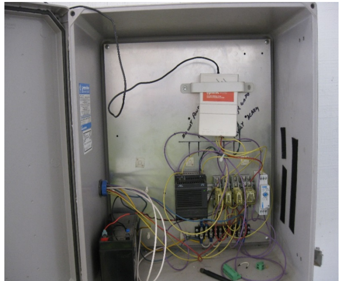
Interior of Instrumentation Panel with RTU
