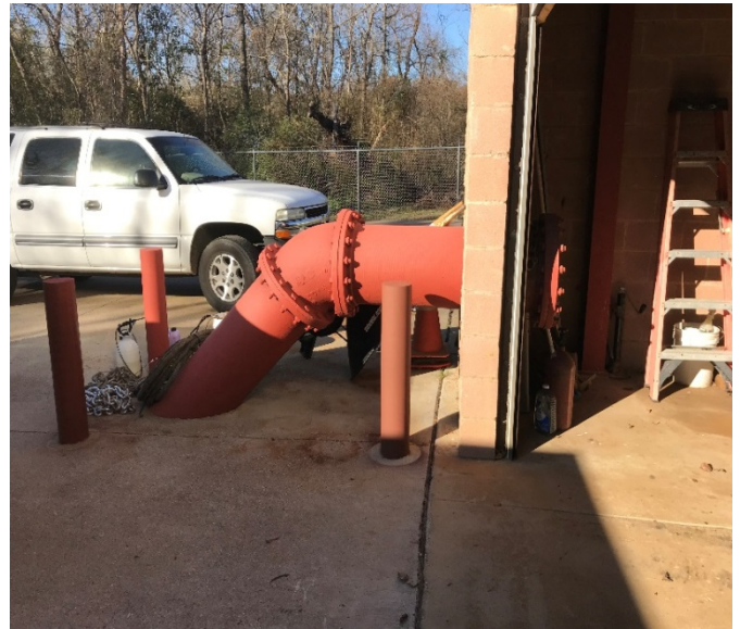
Piping for Future Expansion
