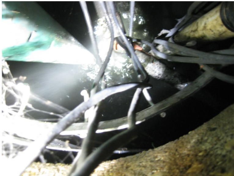
Very Limited Wet Well Visibility
