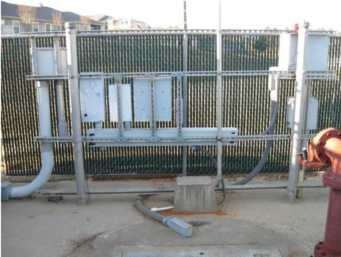
Electrical and Instrumentation Panel Facing Fence and Allowing for Limited Access
