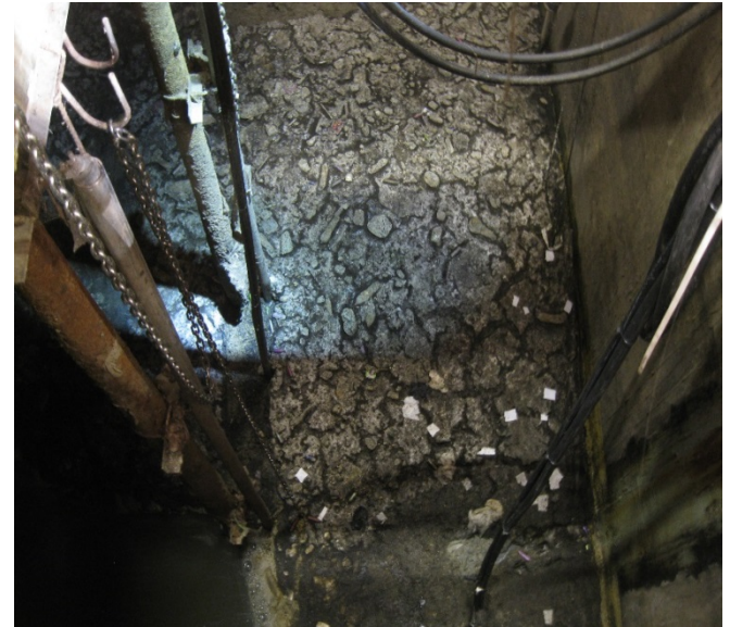
Extensive Debris and Fat, Oils, Grease Deposit Inside Wet Well
