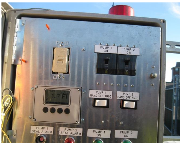
Inside Instrumentation Panel
