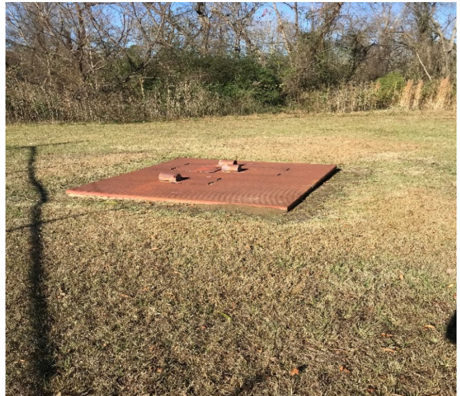
Valve Vault in Backyard. Problems with High Water Levels.
