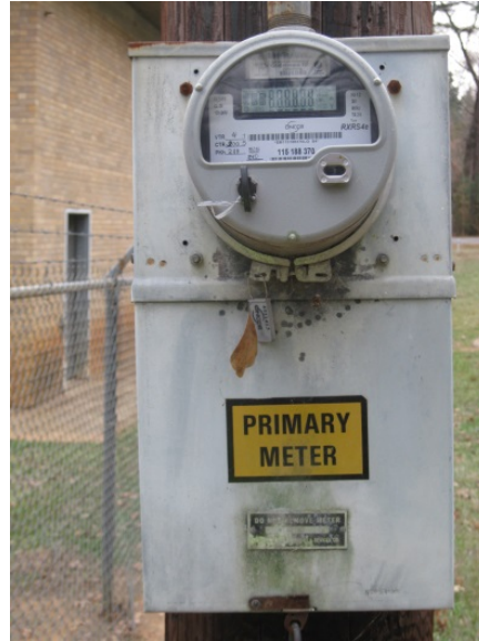
Primary Meter in Fair Condition
