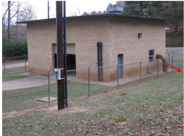
Lower Half of Window Panel Glass Missing on Westside of Building
