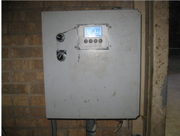
Front of Instrumentation Panel. No Visual or Audible Alarm System Observed On Site
