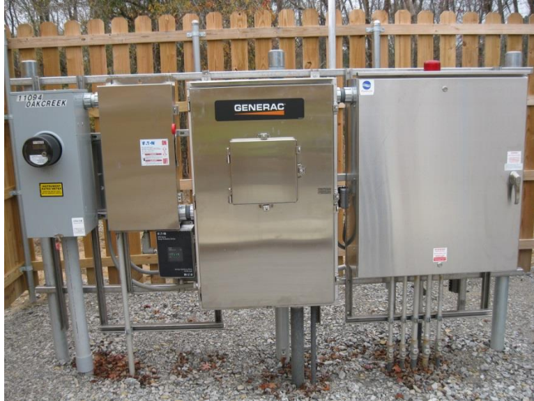
Instrumentation/Electrical Panels in Good Condition
