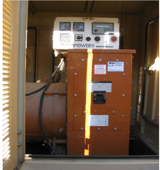
Interior of Generator Enclosure
