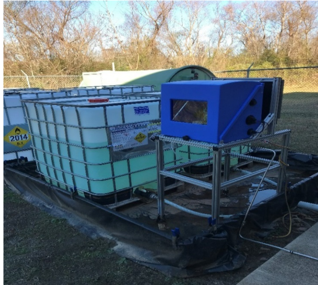
Hydrogen Peroxide Stored On-Site and Used for Odor Control
