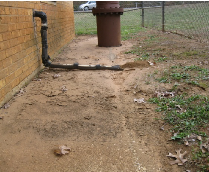
Shallow Foundation Exposure (0"-3") on Westside of Building Allows Drainage Into Building
