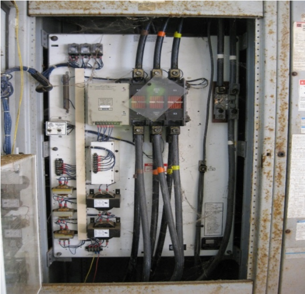
Interior of Generator Control Panel
