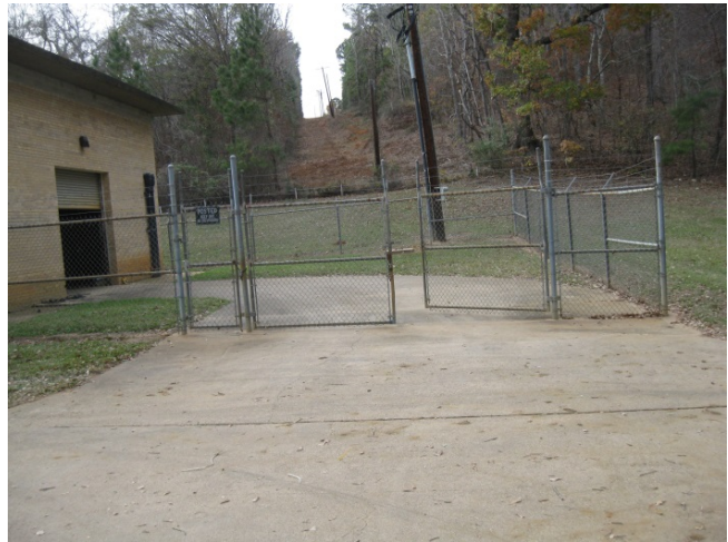
Lift Station Perimeter Fence Facing West. Minor Corrosion Observed.
