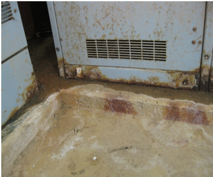
Moisture and External Soil Seepage Around Electric Panel Slab
