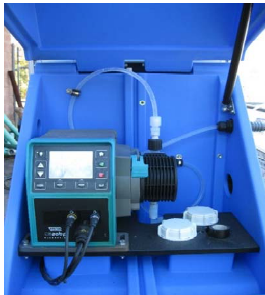
Metering Pump for Hydrogen Peroxide
