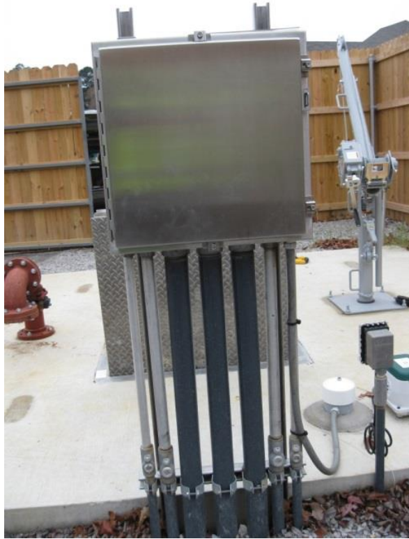
Electrical Panel in Good Condition
