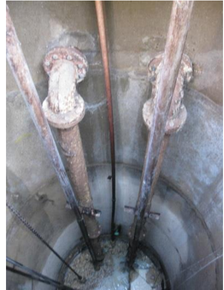
Interior of Wet Well
