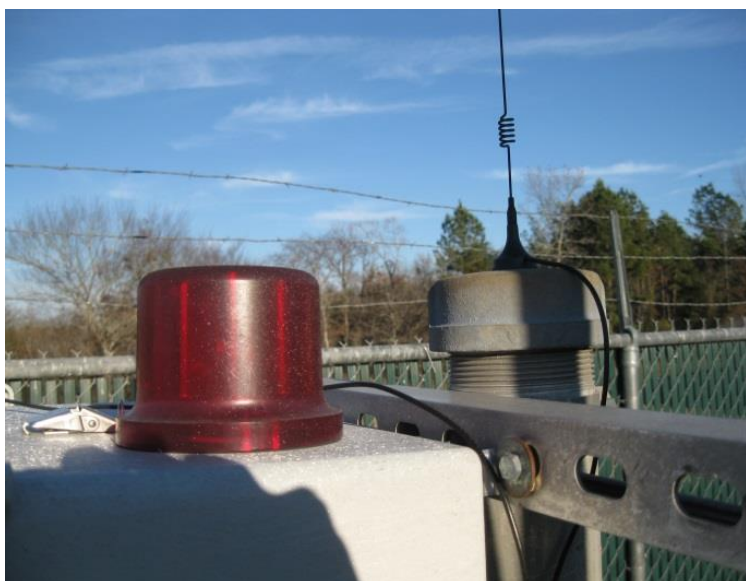
Visual and Sound Alarm on Instrumentation Panel, Antenna Mounted on Conduit Piping
