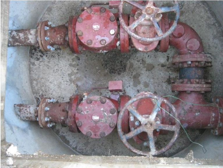
Corrosion on Check Valves
