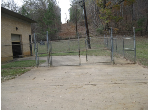
Lift Station Building Adjacent to Steep Natural Ground Facing West. No Flood Protection Measures in Place.
