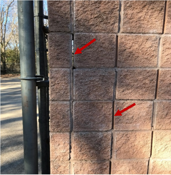
Cracked CMU Wall
