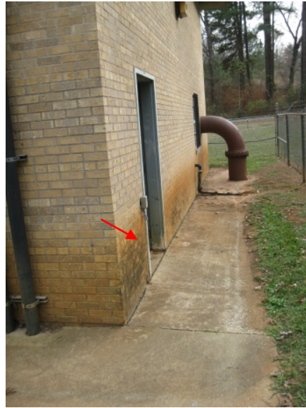
High Water Level Mark on Walls of Building Show Indication of Prior Flooding
