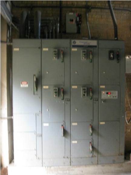
Front of Electrical Panel/Enclosure in Fair Condition
