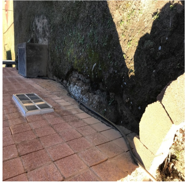
Damaged Exterior Wall
