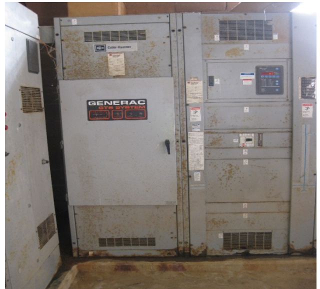
Significant Corrosion on Generator Control Panel
