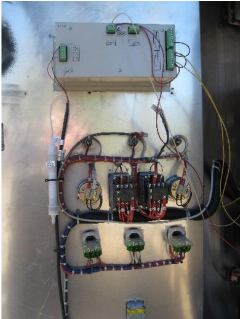
Inside Instrumentation Panel Door
