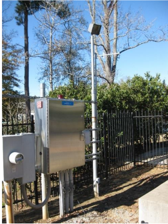
Electrical and Instrumentation Panels in Good Condition
