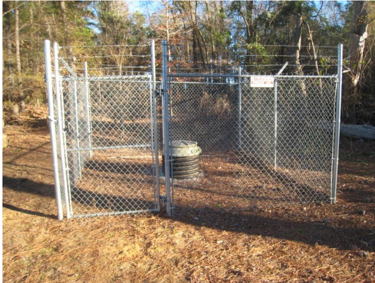
Lift Station Perimeter Fencing and Gate
