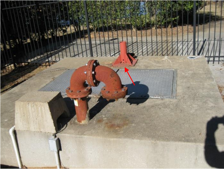
Minimal Corrosion and Peeling on Crane Attachment Fitting
