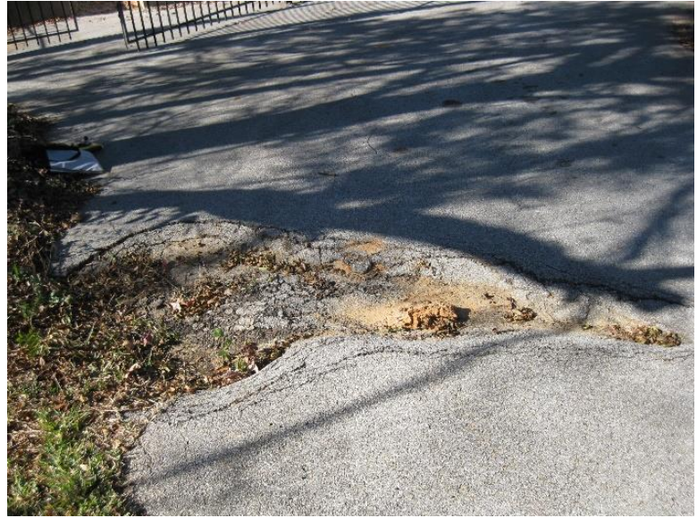
Asphalt Damage on Driveway
