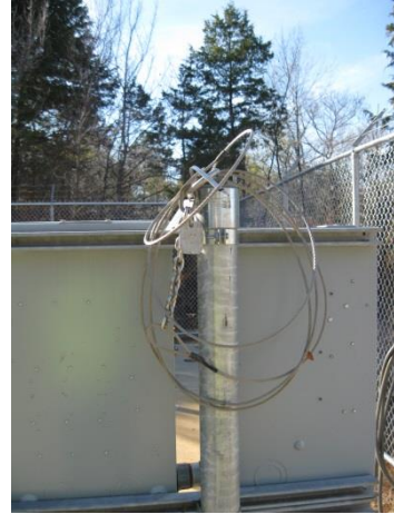
Cable Found Coiled on Instrument Panel Post
