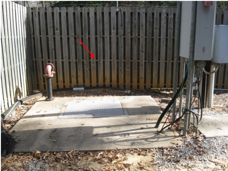
High Storm Water Drainage Mark on Fence; +/- 1-Foot in Areas
