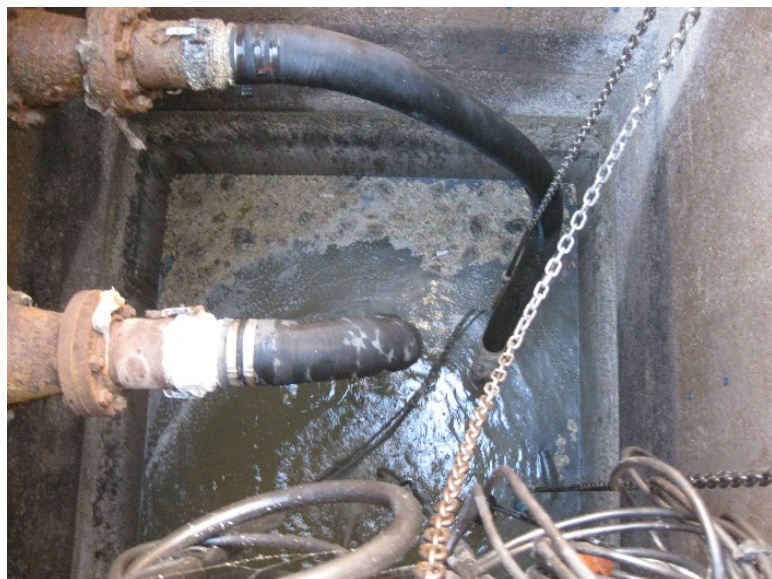
Wet Well Interior With Suction Pipes
