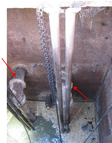
Suction Pipe Shows Signs of Corrosion
