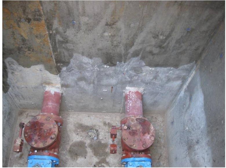
Check Valves in Valve Vault
