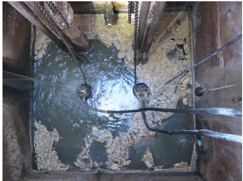
Interior of Wet Well With Riser Pipes and Chain Links for Pumps Visible
