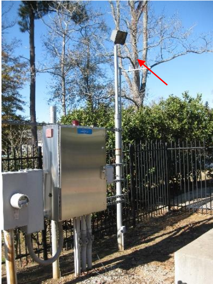
Antenna on Light Pole
