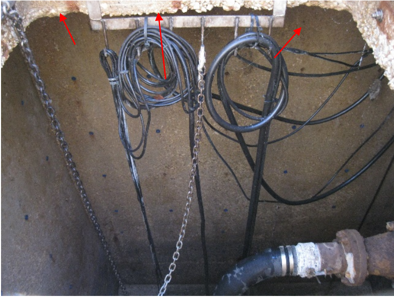
Wet Well Rim Shows Some Deterioration Due To Exposure to Corrosive Environment
