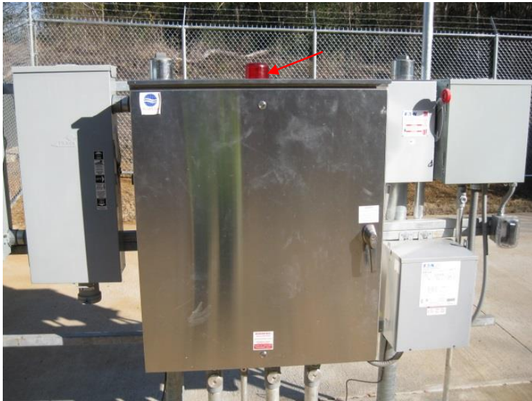
Visual and Sound Alarm on Instrumentation Panel
