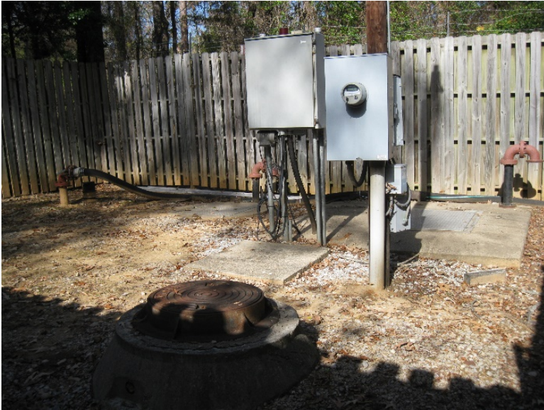
Front of Electrical & Instrumentation Panel
