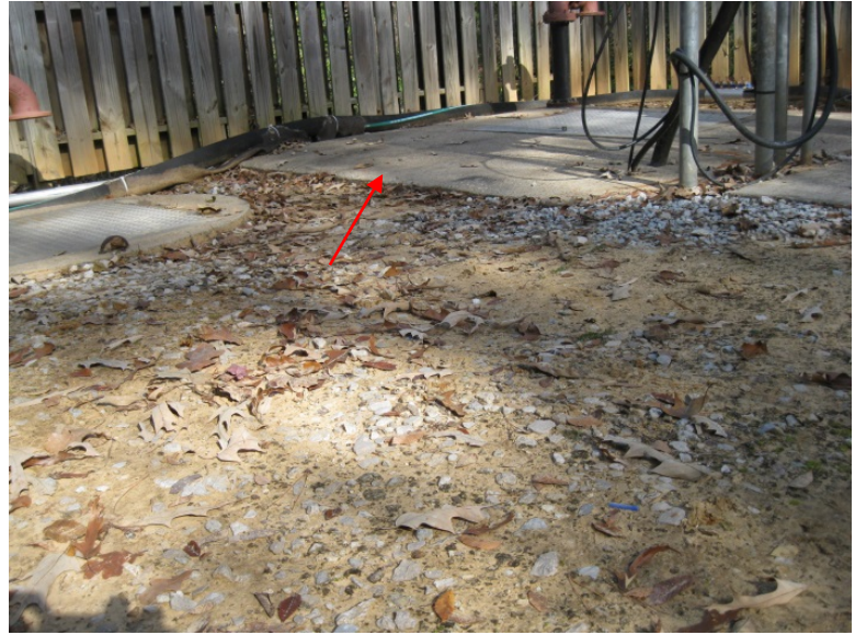
Side of Wet Well Slab Flush With Ground Allowing Drainage onto Slab
