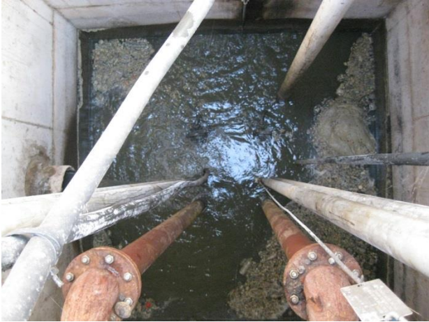
Minor Amount of Oil and Fat Deposits in Wet Well
