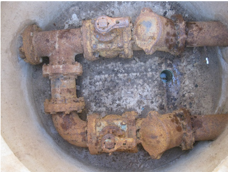
Check Valves with Surface Corrosion
