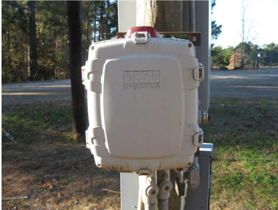
Environmental One Fiberglass Panel With Strobe Light Alarm
