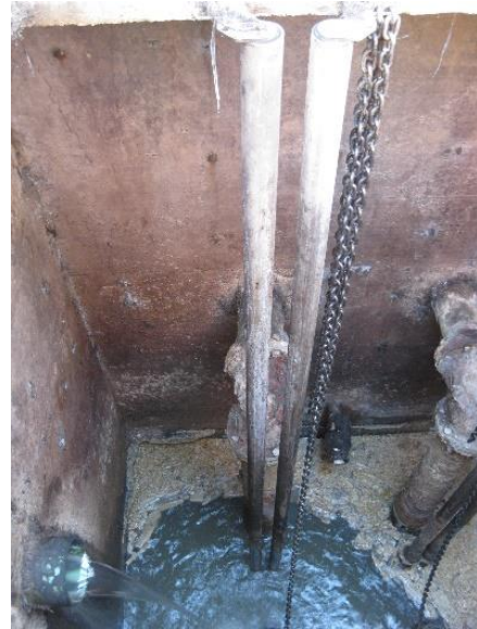
Wet Well Interior
