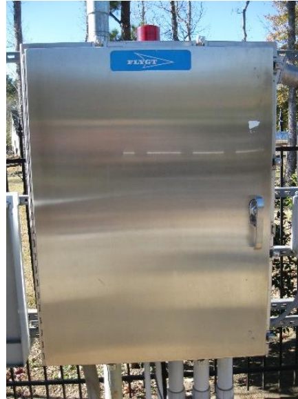
Visual and Sound Alarm on Instrumentation Panel
