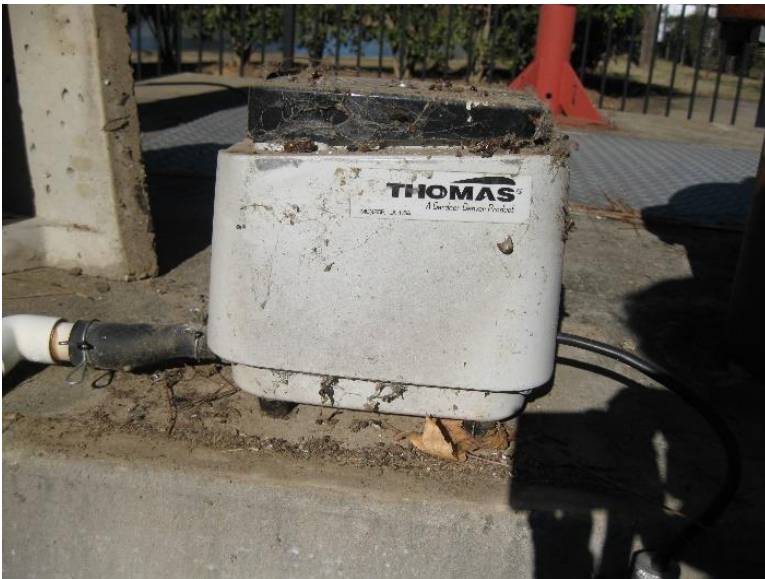
Air Compressor on Slab Below Control Panel For Wet Well Aeration
