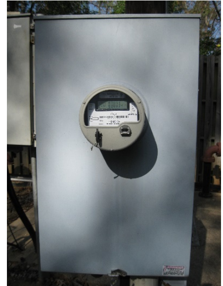
Electric Meter Panel
