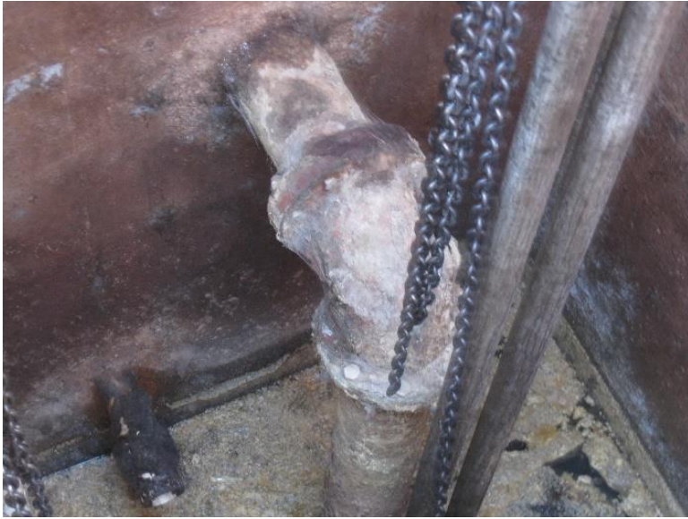
Fitting in Poor Condition in Wet Well
