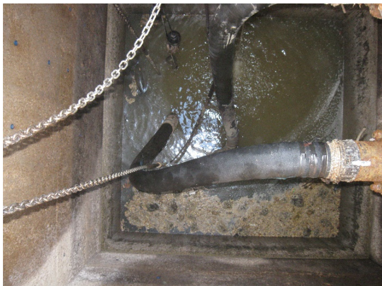
Wet Well Interior with Suction Pipe and Chain Links for Pumps
