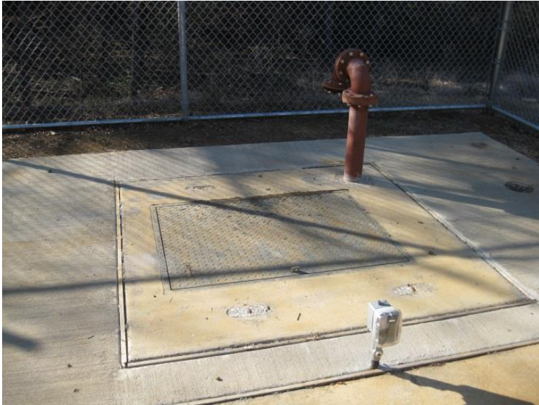
Minor Corrosion on Top Surface of Hatch (1)
