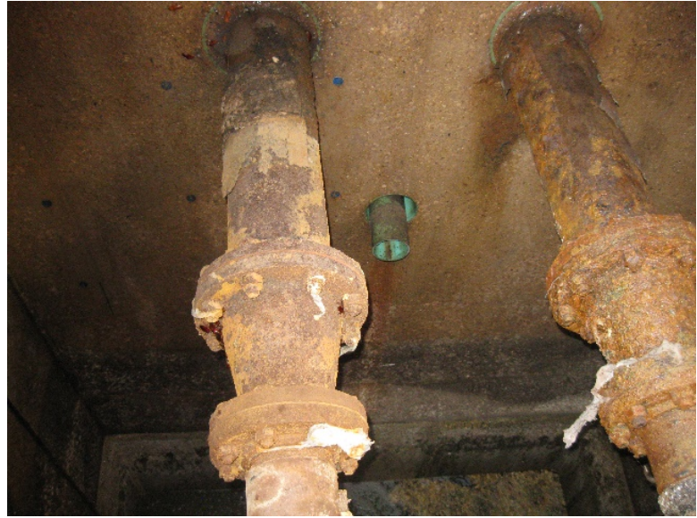
Components in Valve Vault With Corrosion (1)
