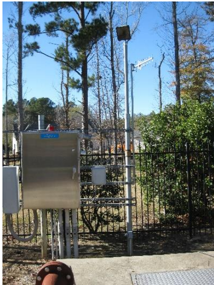
Lift Station Lighting Mounted on Pole. In Need of Maintenance
