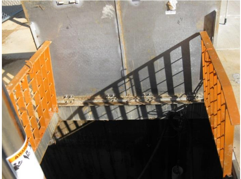
Wet Well Hatch Open
