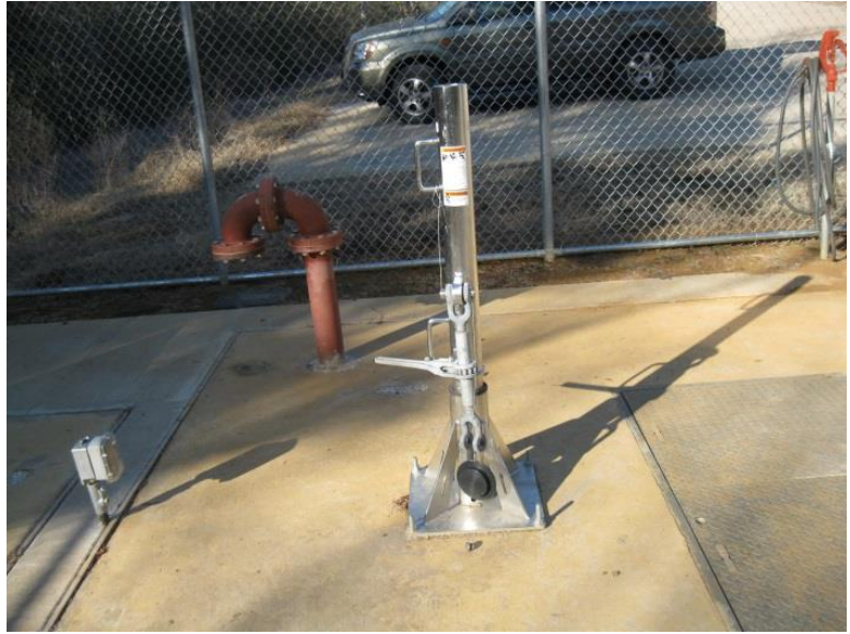
Hoist for Submersible Pumps
