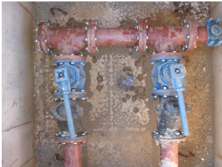
Check Valves in Valve Vault
