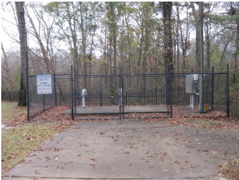
Lift Station Perimeter and Gate
