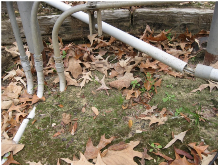
PVC Wire Conduit Not Connected at Fitting
