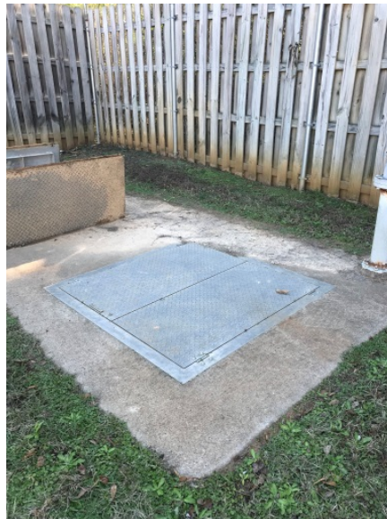
Valve Vault Slab Flush With Natural Ground with Signs of Erosion Around the Slab
