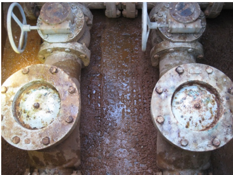
Minor Corrosion on Valves in Valve Vault
