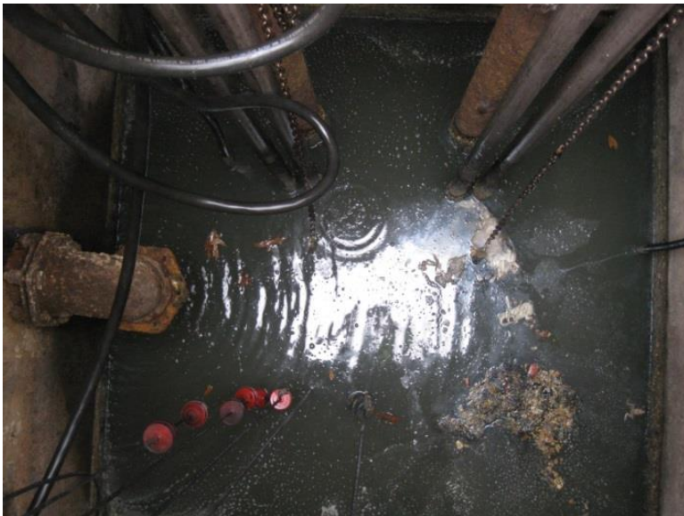
Wet Well Piping Showing Signs of Corrosion
