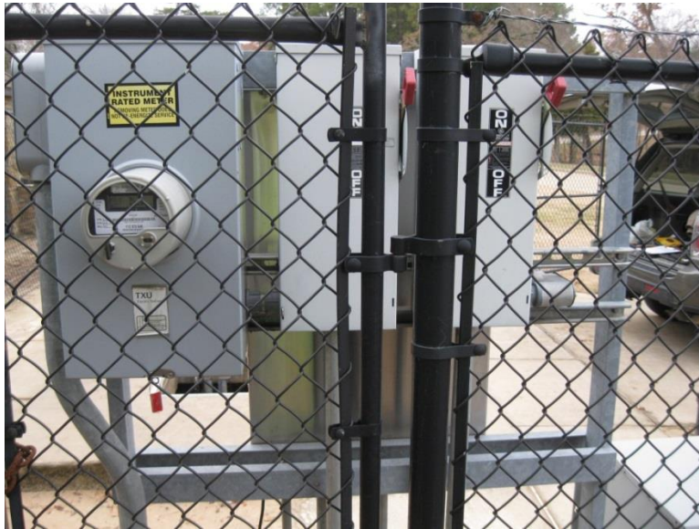
Electrical Panel Facing North
