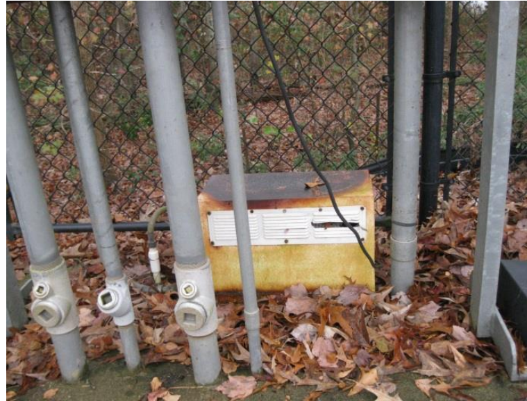
Air Compressor For Wet Well Aeration
