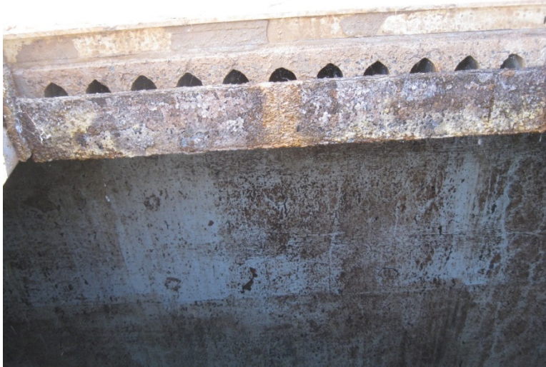
Wet Well Rim Not Coated and Showing Some Corrosion
