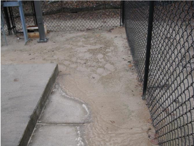
Erosion Silt on Concrete Surface Facing East
