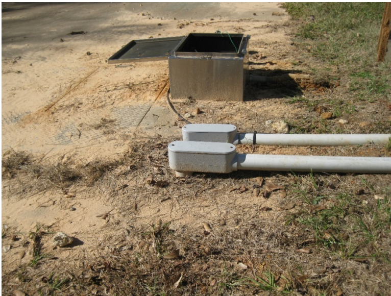
Abandoned Electrical Junction Box on Wet Well Slab
