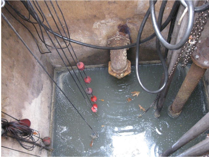
Wet Well Interior
