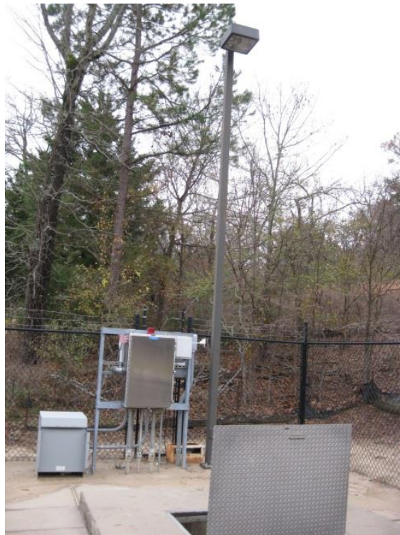
Electrical Panel Mounted on Vertical Frame
