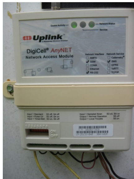
Uplink RTU Inside Instrumentation Panel Door
