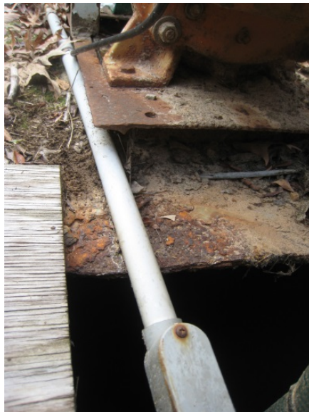
Pump Frames Corroded
