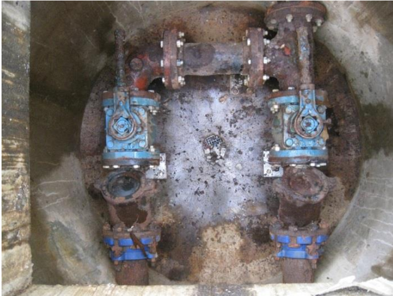
Check Valves With Significant Corrosion
