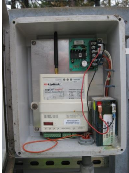
Uplink RTU Inside Instrumentation Panel
