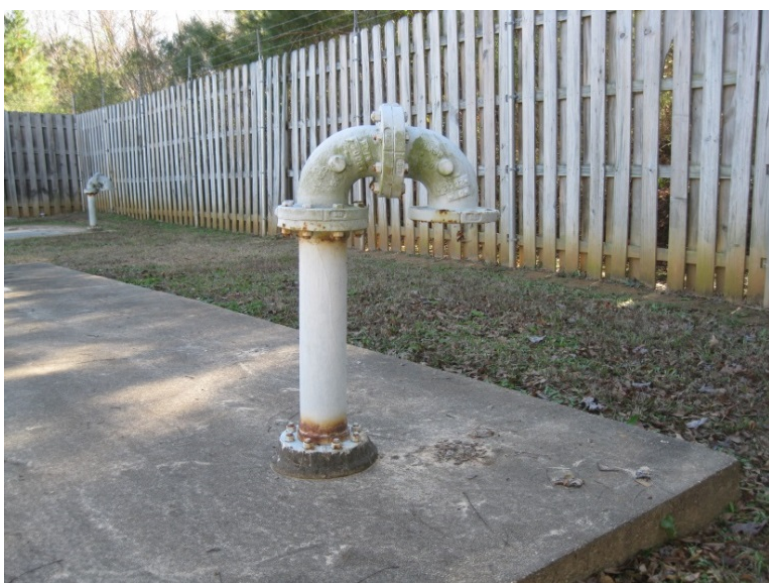
Minor Corrosion on Ventilation Pipe
