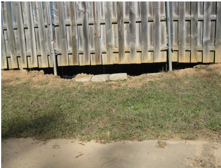
Erosion Around Fencing Facing South
