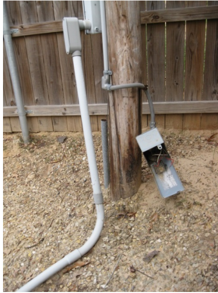
Open Exposed Junction Box at Base of Service Pole
