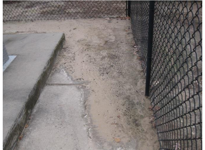
Erosion Silt on Concrete Surface Facing West
