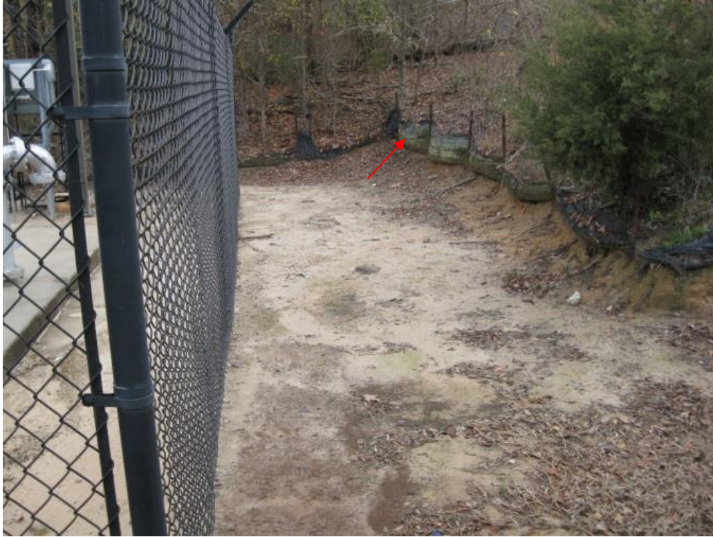
Uphill Slope Behind Lift Station Held Back By Fence. Fence in Poor Condition but Not City Property to Allow For Repair and Maintenance
