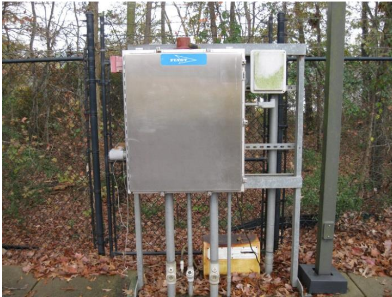
Front of Instrumentation Panel
