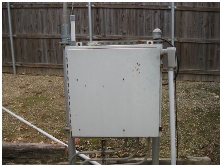
Instrumentation Panel With Corrosion
