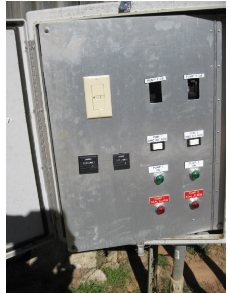
Electric Panel Interior
