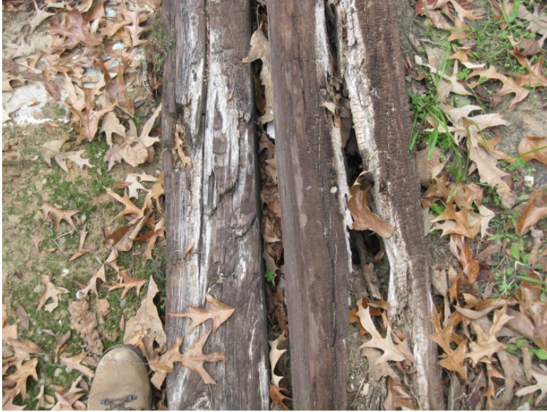
Railroad Tie Retaining Wall Deteriorated (1)
