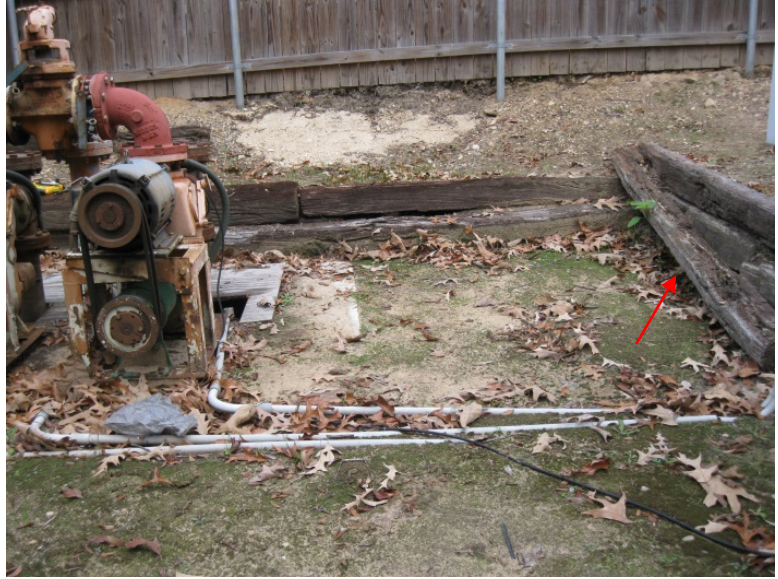
Railroad Tie Retaining Wall Deteriorated (2)
