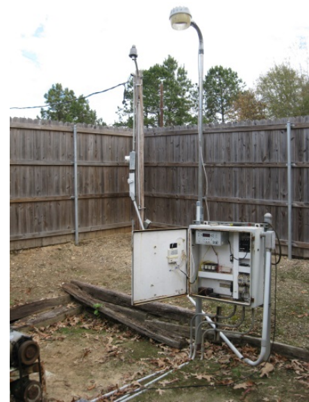
Lift Station Perimeter Facing South. Light Bulbs Broken in Both Lights On Site
