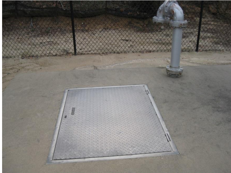
Wet Well Hatch
