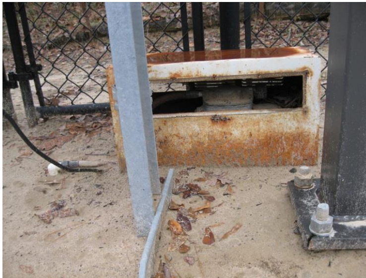
Air Compressor in Cover- Signs of Corrosion
