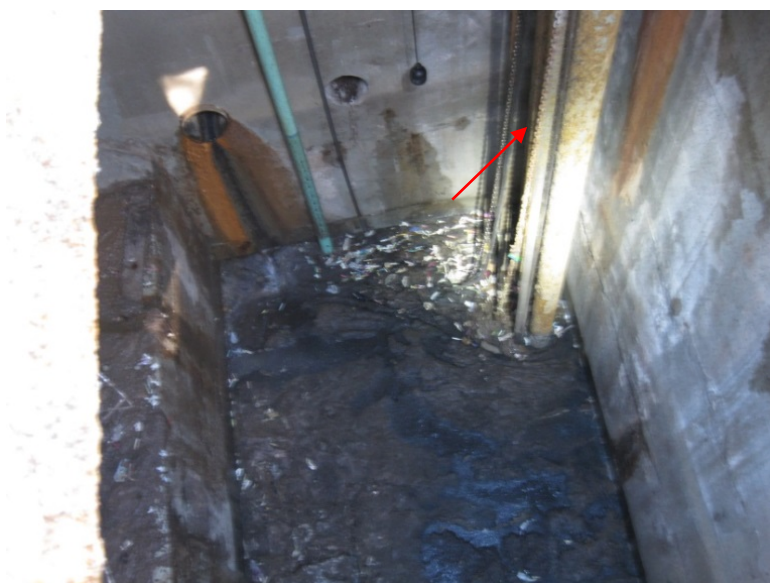
Corrosion on Chains and Rails
