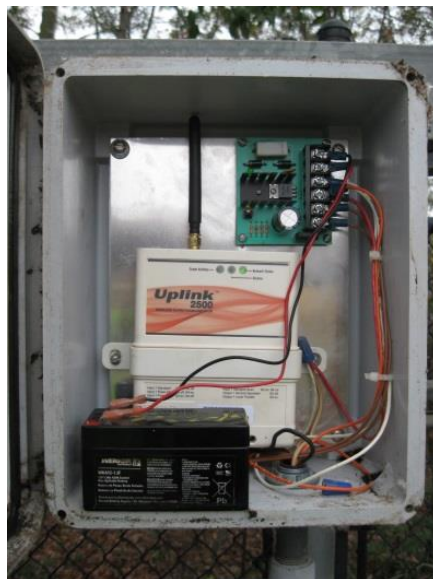
Uplink RTU Inside Instrumentation Panel
