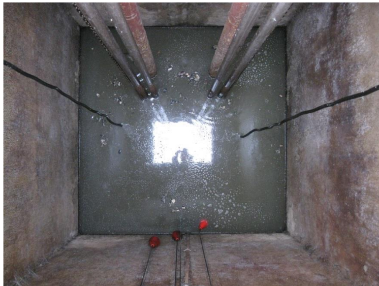
Wet Well Interior
