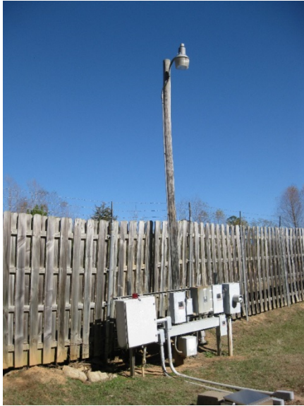
Electrical and Instrumentation Panel Facing South
