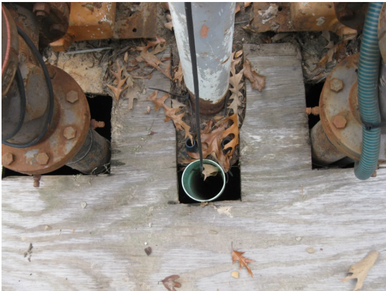
Wet Well Top Covered With Wooden Board. Openings Allow I/I Into Wet Well
