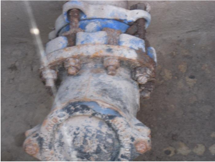
Bolts on Check Valve Showing Some Corrosion
