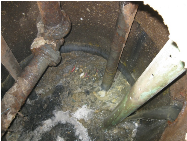
Significant Debris in Wet Well
