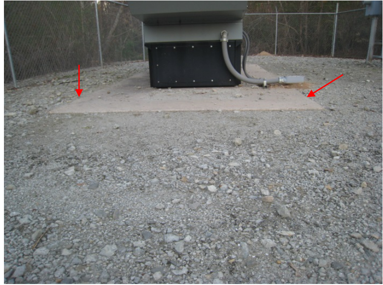
Generator Slab Flush With Ground, Allows Water to Come into Contact With Generator Base
