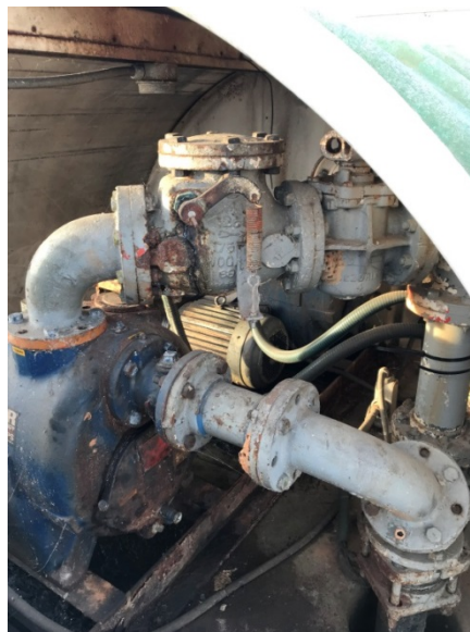
Pumps, Suction Pipe and Fittings Show Some Corrosion
