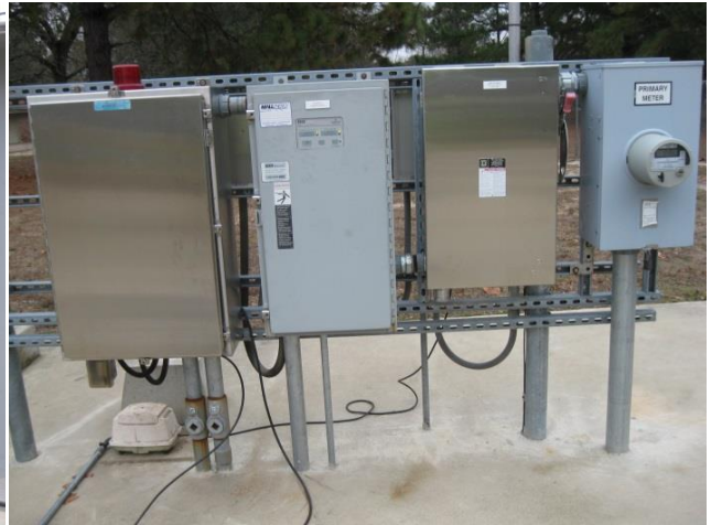
Instrumentation Panel in Good Condition
