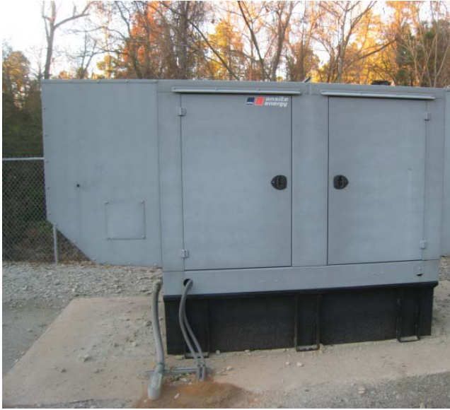
Front of Generator
