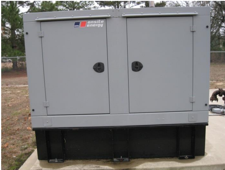
Front of Generator
