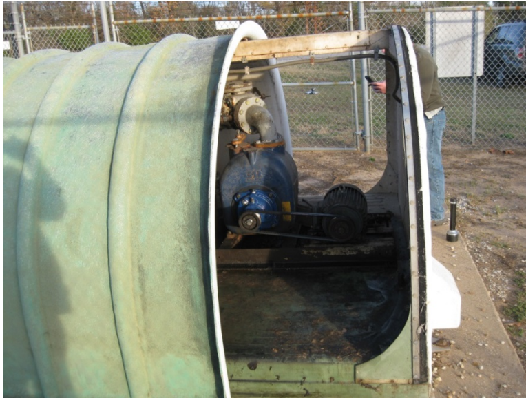
Valves Difficult to Access if Dog House Cannot Be Completely Opened
