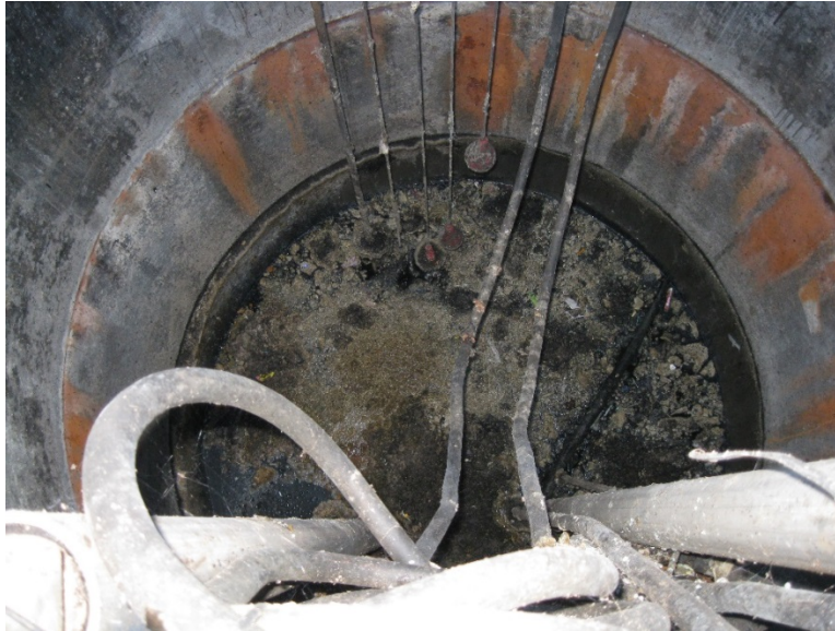
Fat, Oil and Grease Deposits on Wet Well
