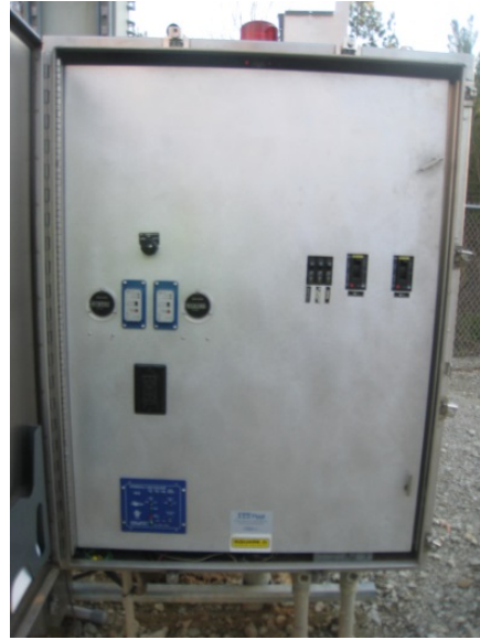
Inside of Instrumentation Panel (1)
