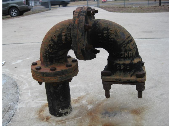
Ventilation Pipe Shows Significant Corrosion
