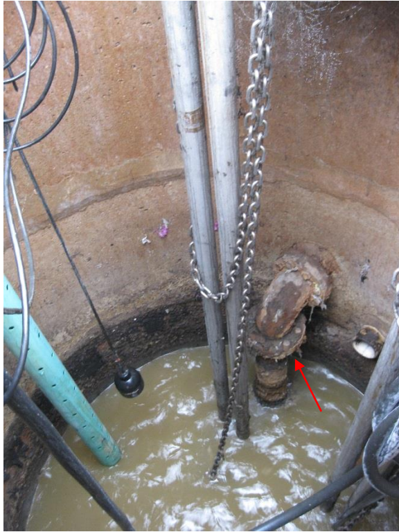
Suction Pipe Shows Signs of Corrosion
