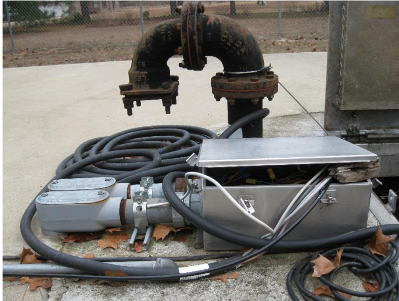
Electric Junction Box Near Wet Well
