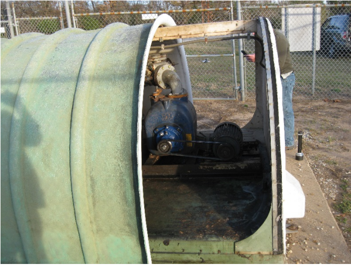
Lift Station Dog House Front- Facing East
