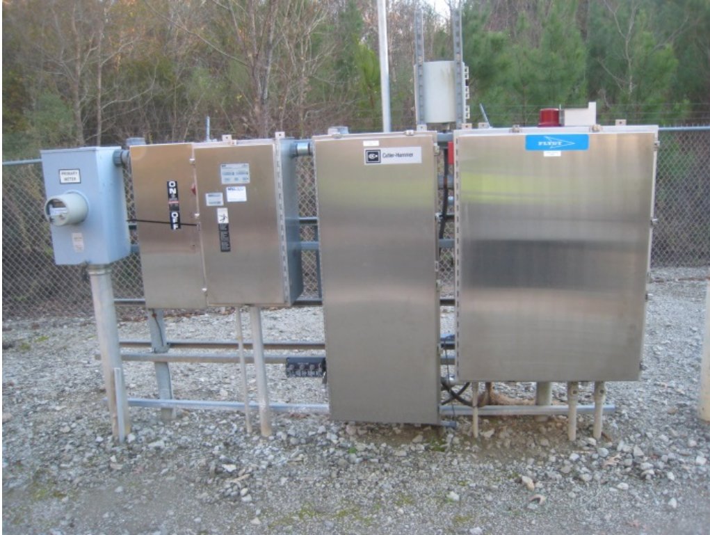
Instrumentation Panel Facing South
