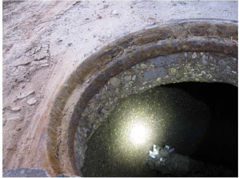
Wet Well Rim Concrete Deterioration
