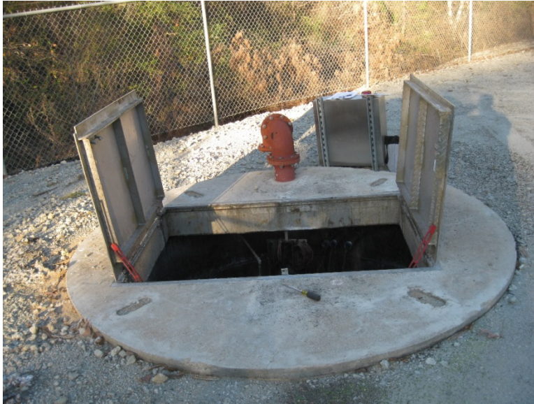
Exterior of Wet Well With Hatch Open and Vent Pipe for Wet Well
