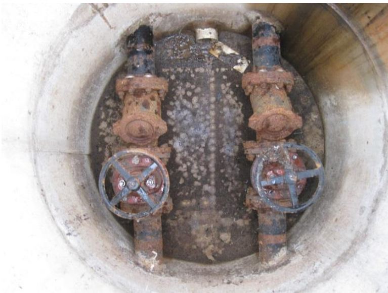
Check Valves With Significant Corrosion
