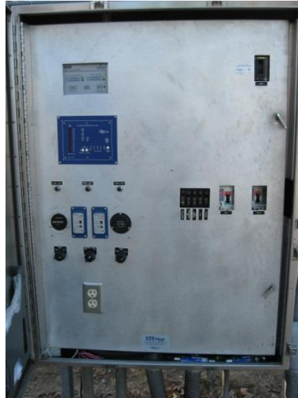
Inside of Instrumentation Panel (1)
