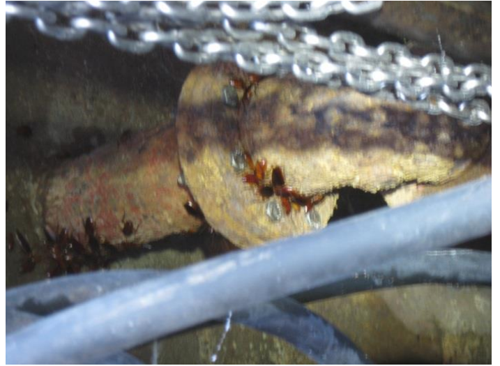
Riser Pipe in Wet Well- Corroded
