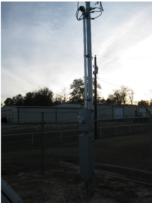
Electrical and Instrumentation Panel Mounted on Pole- Facing Southwest
