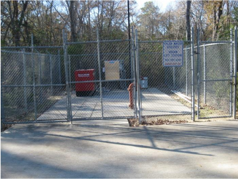
Lift Station Perimeter Facing West
