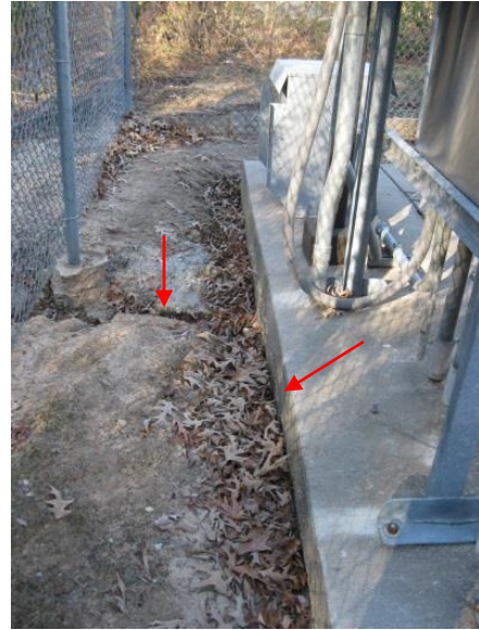
Erosion Near West Fence
