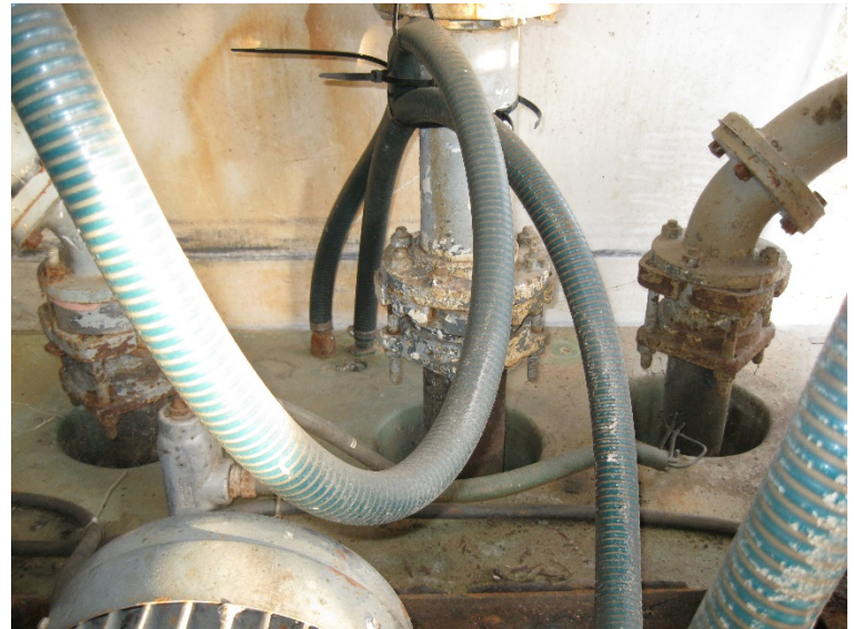
Gaps Visible At Points Where Suction Pipes Enter Wet Well
