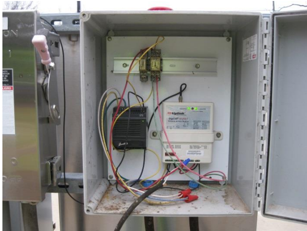
Uplink RTU in Good Condition
