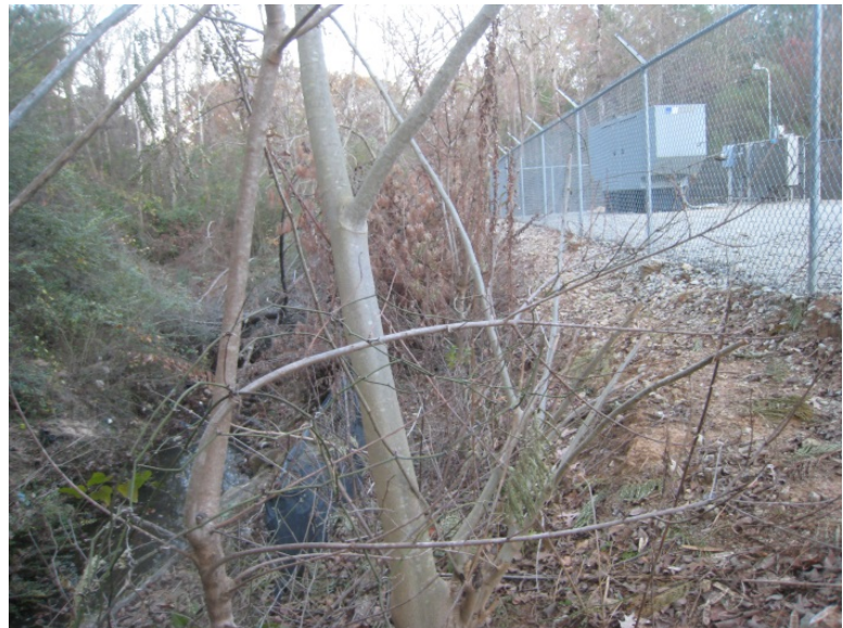
Flooding from Adjacent Creek Could Cause I/I Into Wet Well In Future
