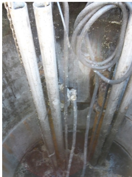
Debris at Top of Wet Well Indicate Previous Overflow Conditions
