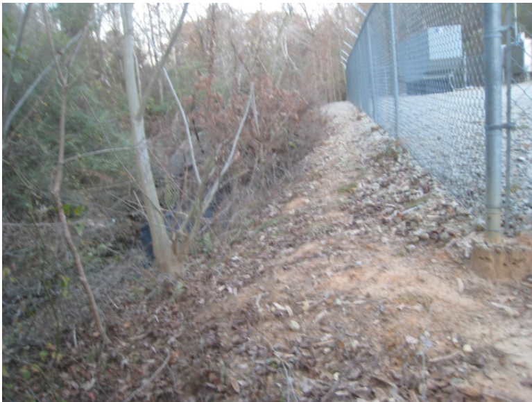
Erosion Exposing Fence Pole Piers
