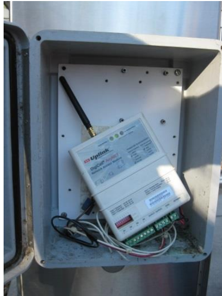
Uplink RTU Inside Instrumentation Panel
