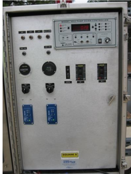
Inside of Instrumentation Panel (1)
