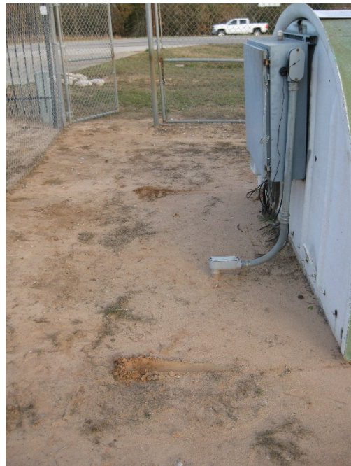
Dog House Roof Beam Corrosion
