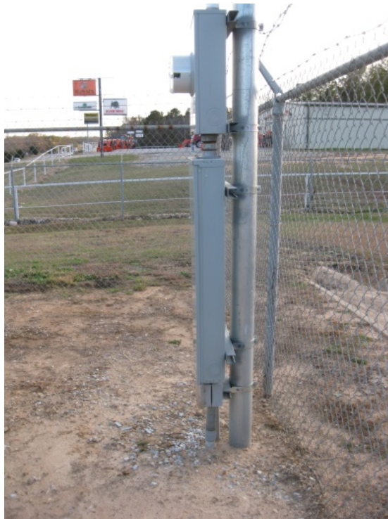
Electrical Meter Mounted On Pole
