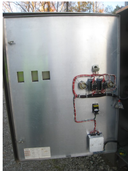
Inside of Instrumentation Panel Door
