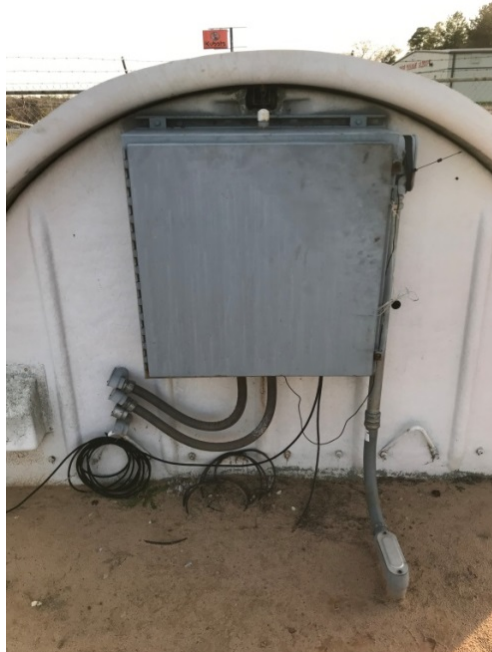
Electrical and Instrumentation Panel Mounted on Dog House Rear Wall
