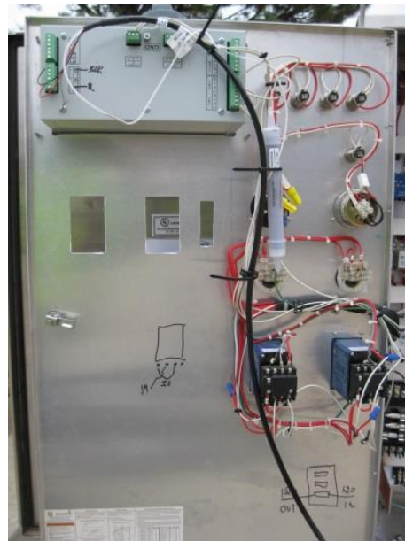
Inside of Instrumentation Panel Door
