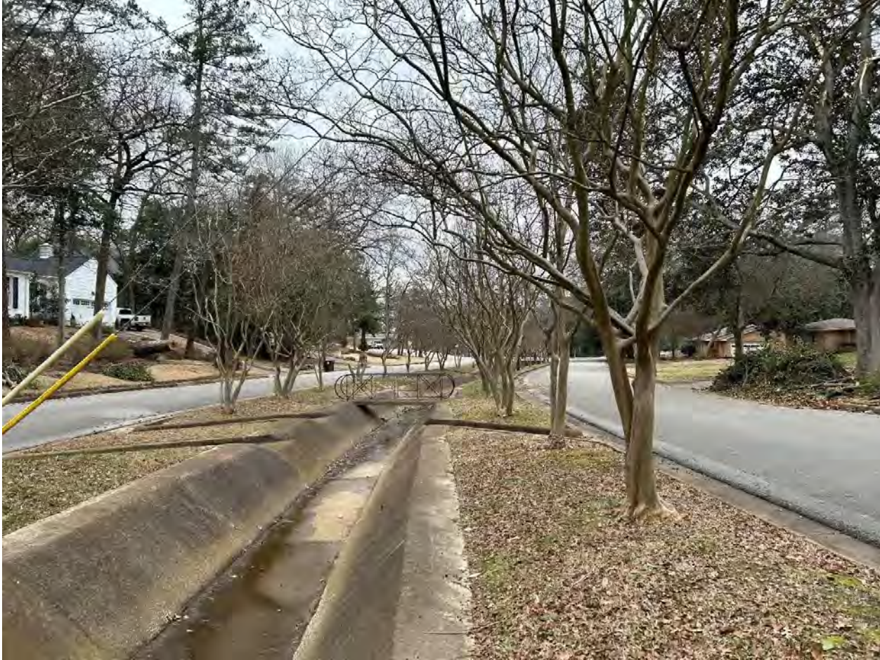
Photo 18. The drainage canal with pedestrian bridge (Resource 139652) in the 3500 block of Woodbine Boulevard. Camera facing north.
