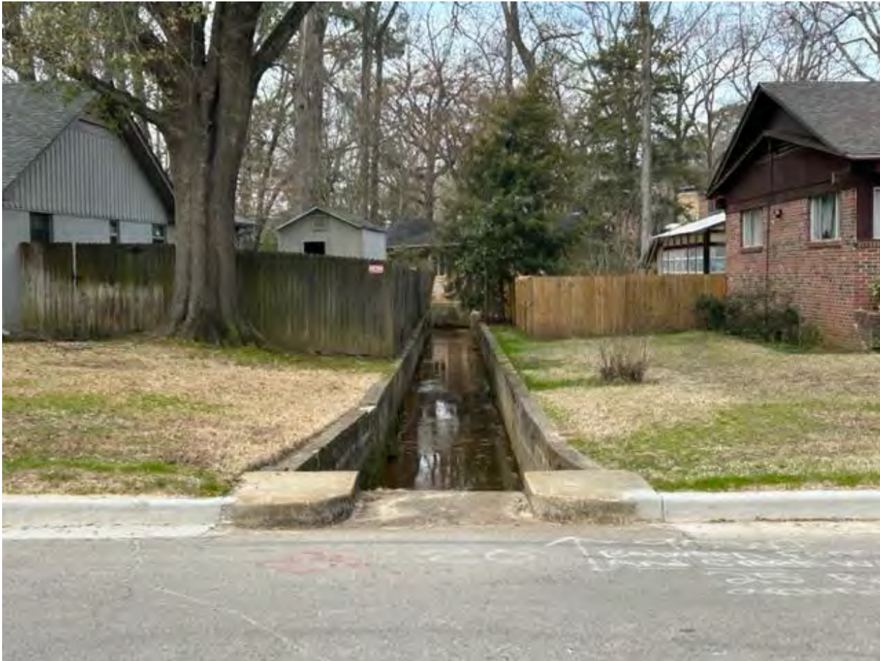
Photo 19. Concrete lined drainage canal (Resource 139655) in the 3700 block of Fry Avenue. Camera facing west.
